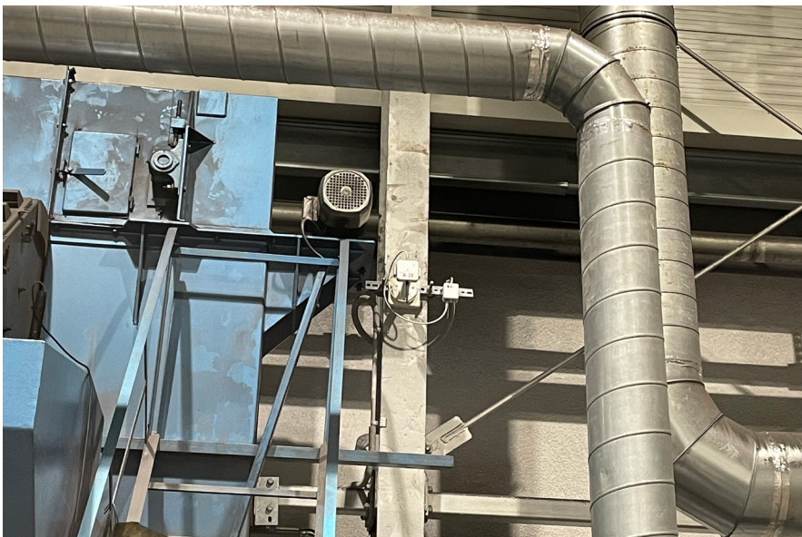
The installation of Sewio anchors by the gate and in between the metallic constructions.
