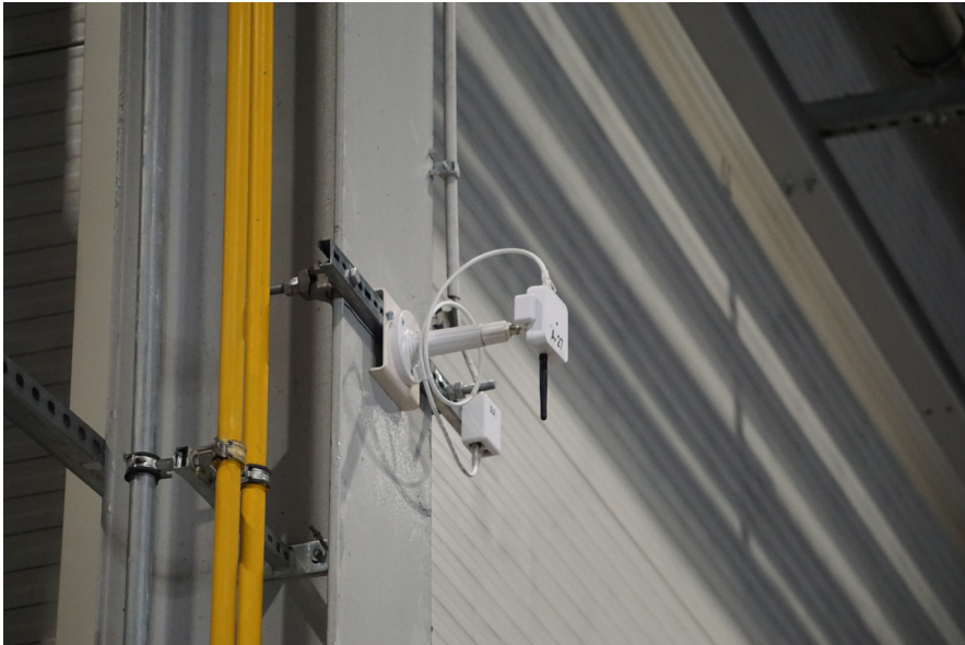
The installation of Sewio anchors by the gate and in between the metallic constructions.
