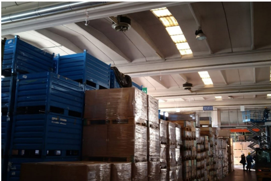
Detail of the anchors installed in the central row of the warehouse.
