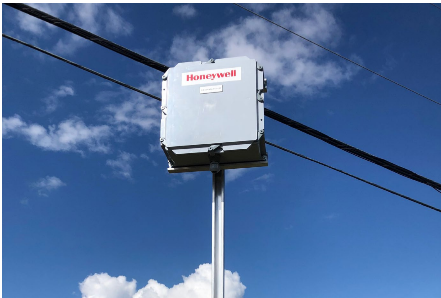
UWB anchor (signal receiver) installed on the post.
