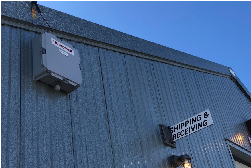
UWB anchor (signal receiver) mounted on one of the halls.
